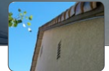
Discrete wiring under soffit
